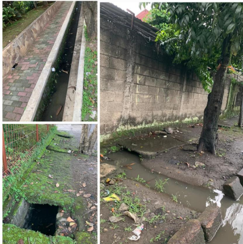
Figure 2. Existing condition of the drainage channel on Jalan Raya Karadenan Source: Research documentation, 2026
